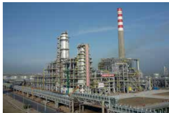
Project: OGD III 3rd NGL Project Country: Abu Dhabi Client: Adnoc UAE Engineering: Bechtel USA/UK Project: AGD II - ASAB Gas Development Phase 2 Country: Abu Dhabi Client: Gasco Engineering: Bechtel USA/UK
