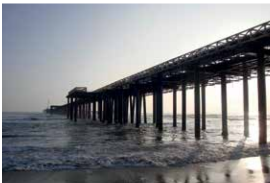
Project: Pampa Melchorita Country: Peru Client: PERU LNG – a consortium led by Hunt Oil (USA) with partners Repsol YPF (Spain), SK Energy (South Korea) and Marubeni (Japan) Engineering: CDB Melchorita – a consortium of Saipem (France), Jan de Nul (Belgium) and Norberto Odebrecht (Brasil)
